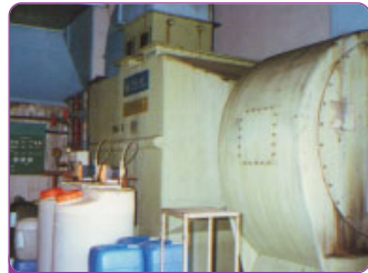
Packed Tower Scrubbers 1
